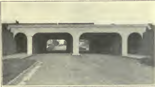
FIG. 275. TRACK ELEVATION. Reinforced concrete bridge of the Illinois Central Railroad at 71st Street.
